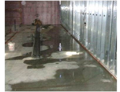
FIGURE 2 – Construction site moisture.
