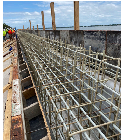
Project designed by Johnson, Mirmiran & Thompson (JMT), with repairs completed by Gulfstream Construction (general contractor) and Palmetto Gunite (subcontractor).
